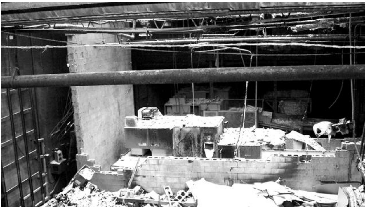
Figure 3: Collapsed firewall between lines 403 and 405 [CSB 38]
