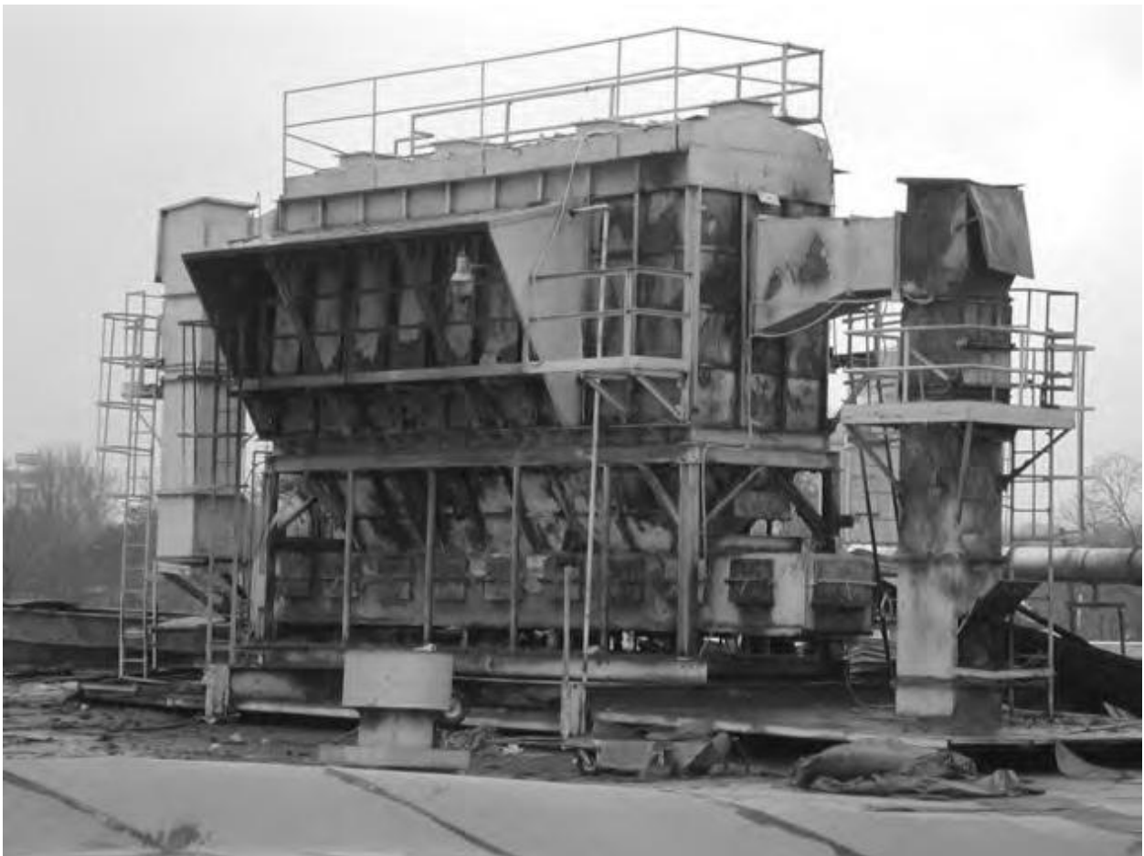
Figure 2: Fire damage to line 405 baghouse [CSB 35]
